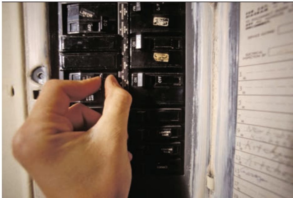
If you have to flip a breaker every time you flip flapjacks on your electric griddle, it's a good idea to have your home wiring inspected and to make the necessary upgrades.
